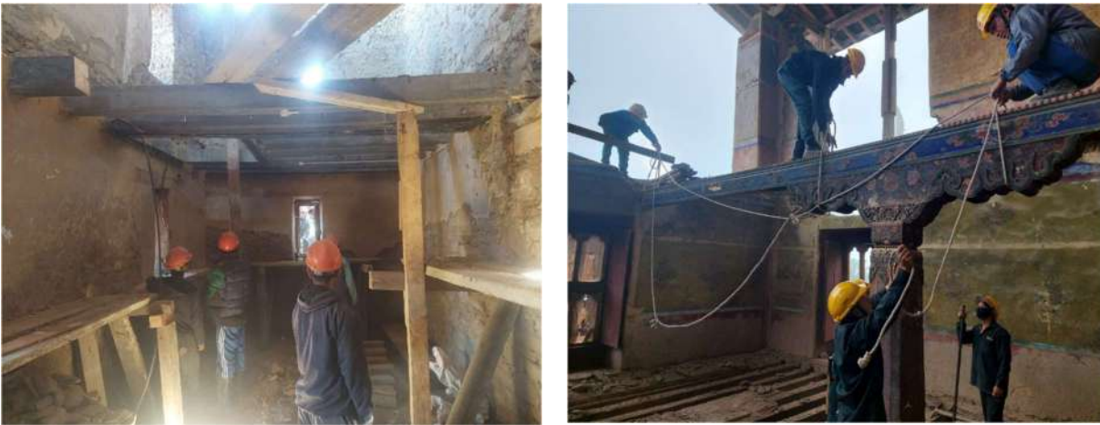
Figure 13: (a) Removal of Cham from stone wall (b) Removal of Dhung along with Zhu (capital) from stone masonry
