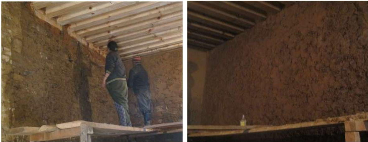
Figure 31: Wetting of wall surface with scaffolding (left) and First layer of wall plaster- Bjidhen (right)
