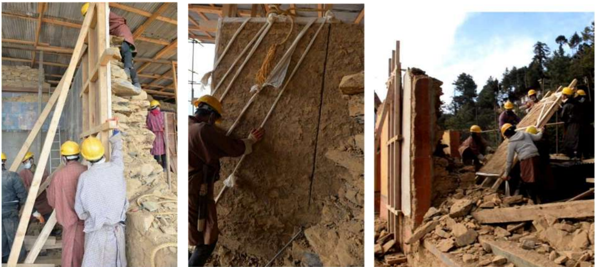
Figure 7: Erection of panel (left), Additional support to the frame and mural (middle) and detached mural with the panel (right)
