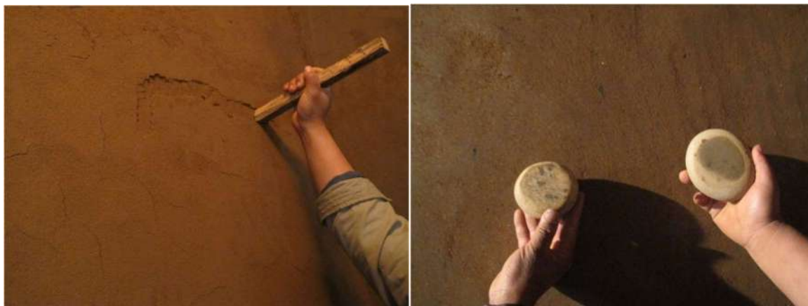
Figure 32: Removal of entrapped air (left) and rubbing the wall plaster using a river stone with flat surface (right)
