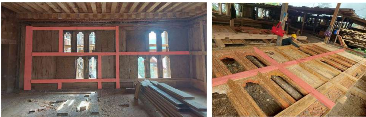
Figure 35: The orange-colored timber elements shows the retained timber components of a Rabsey
