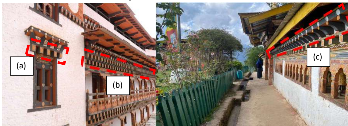
Figure 45: (a) Single Bogh layer, (b) double Bogh layer, (c) Phuto boow with Phakhep
