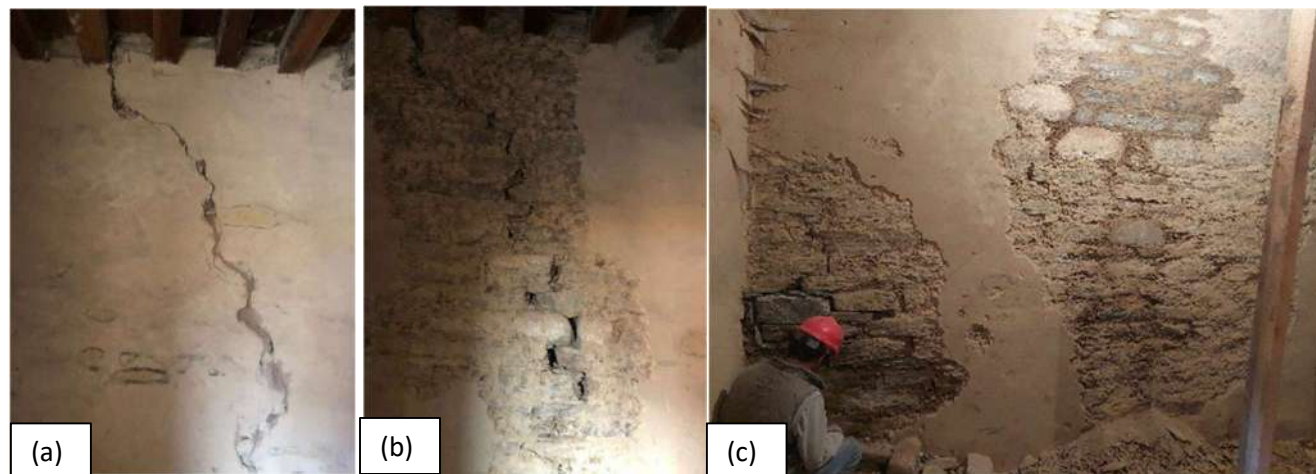
Figure 28: (a) Crack originating from Cham (b) removal of plasters and (c) Stone stitching of wall
