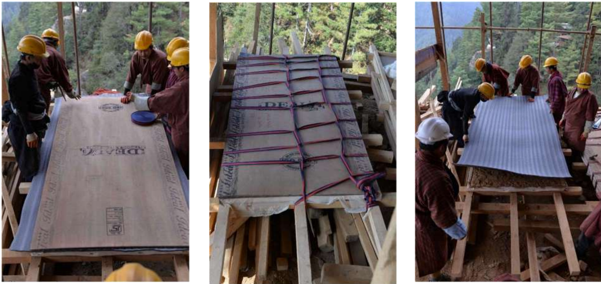
Figure 8: Foam on detached mural (Left), Plywood sheet added (Middle), Completed form (Right)
