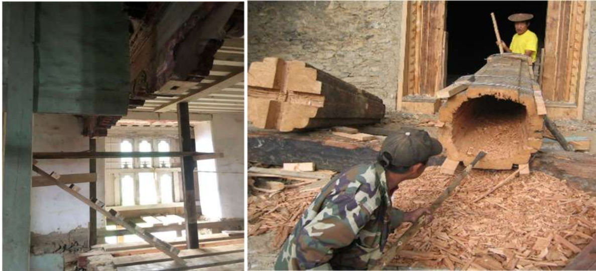
Figure 44: Propping to remove the Kachen (Left) and coring of the inner core of Kachen (right)
