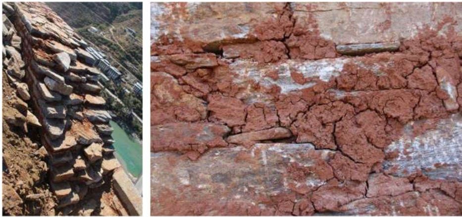
Figure 26: (a) Proper laying of stones (b) The mud mortar with undesirable shrinkage
