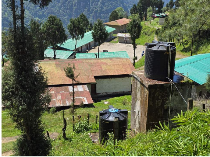
2 Sintex Tanks at Gasa Primary School
