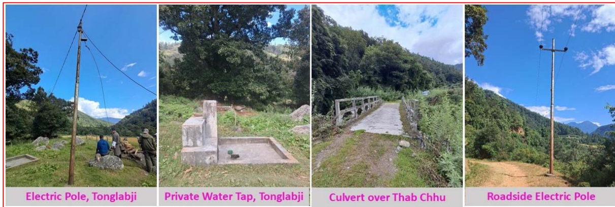
Figure 44: Photographs of Utilities and Culvert over Thab Chhu stream that are likely to be damaged during excavation works (Source: Field survey, October 2025)
