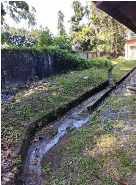
Collapsed Drain inside Army Camp
