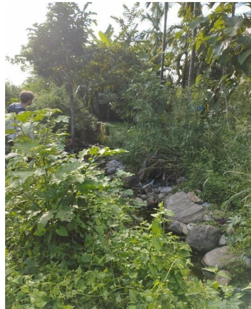
Collapsed Drain at the end of the AWP drain
