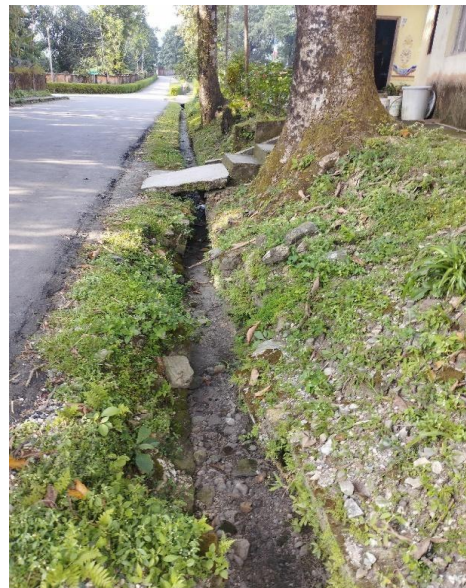
Collapsed Drain near Army Camp
