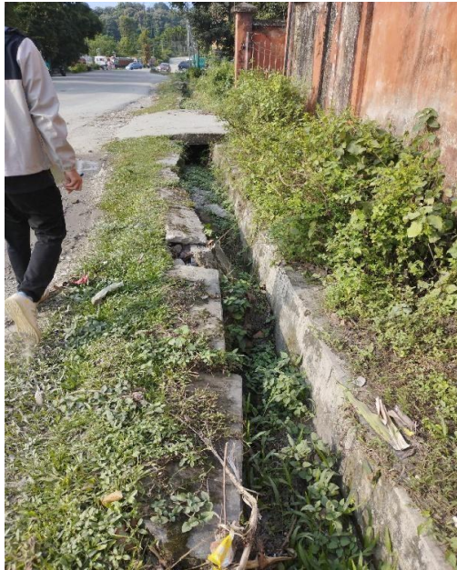
Collapsed Drain near Checkpost
