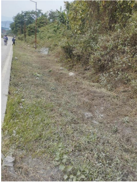
Damaged Drain at Pasakha Industrial State
