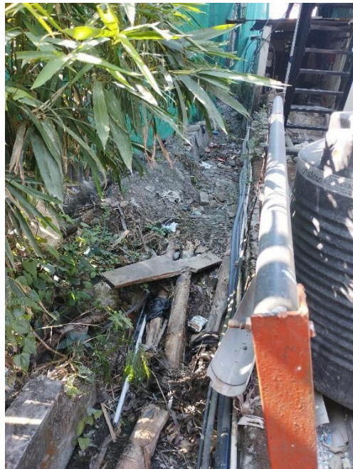
Damaged Drain behind Druk Petroleum
