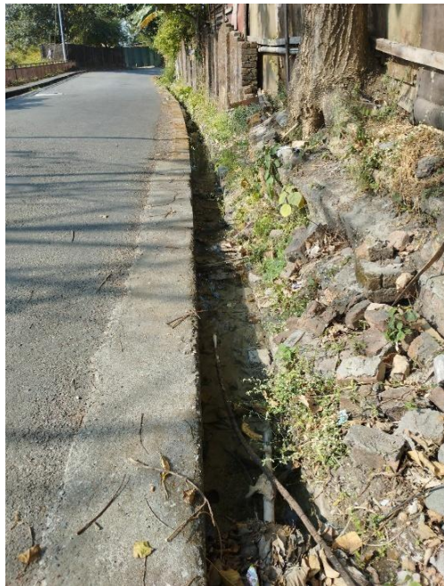
Damaged Drain below Bhutan Packaging Industry
