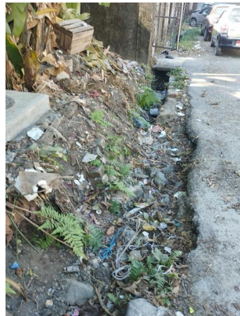
Damaged Drain behind FCB
