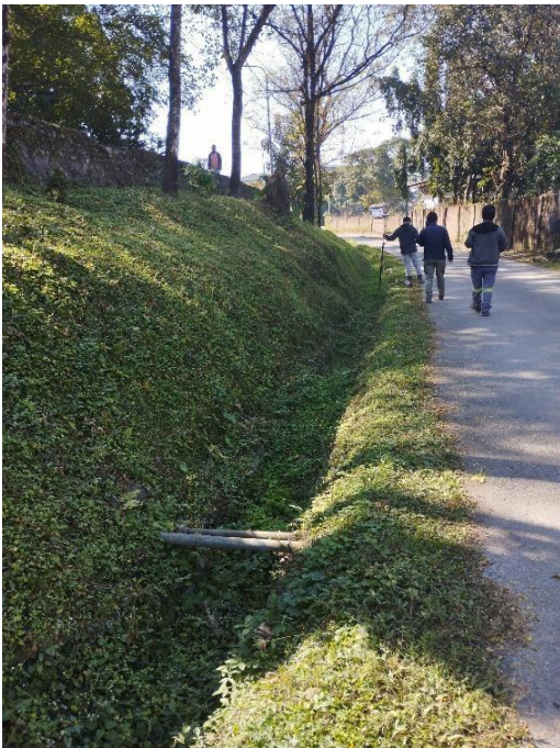
Damaged Drain outside Army Camp
