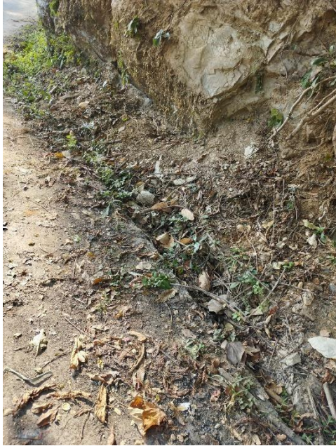
Blocked Drain at Kabrayter
