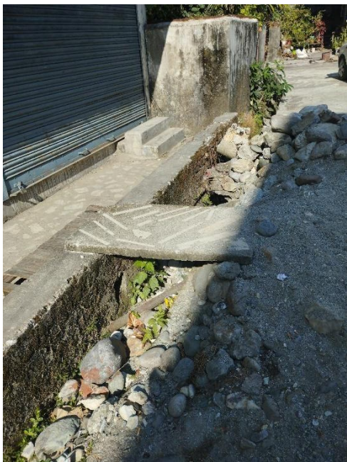
Damaged Drain above PSA ground
