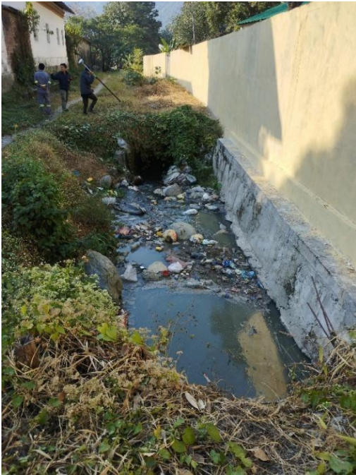
Damaged drain near the terminal
