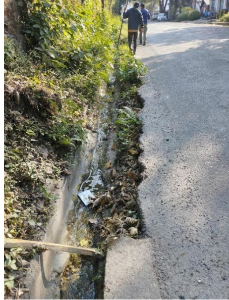
Damaged Drain below Hospital
