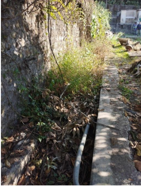
Blocked Drain near School (PRHSS)
