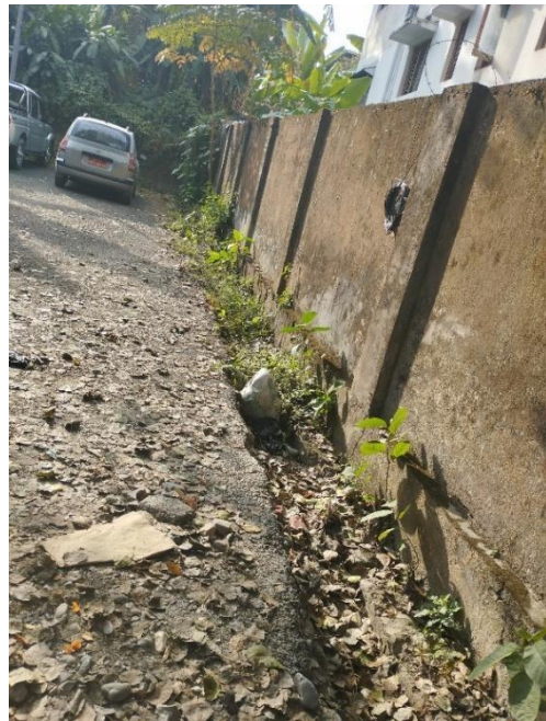
Damaged drain inside Thomde Parking
