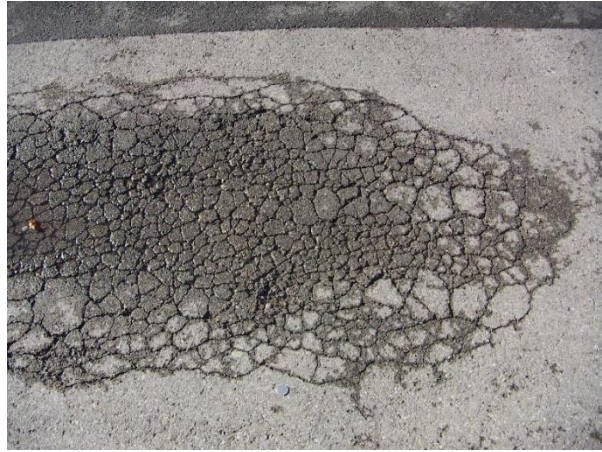
Figure 43: Block cracking and alligator cracking on road surface
