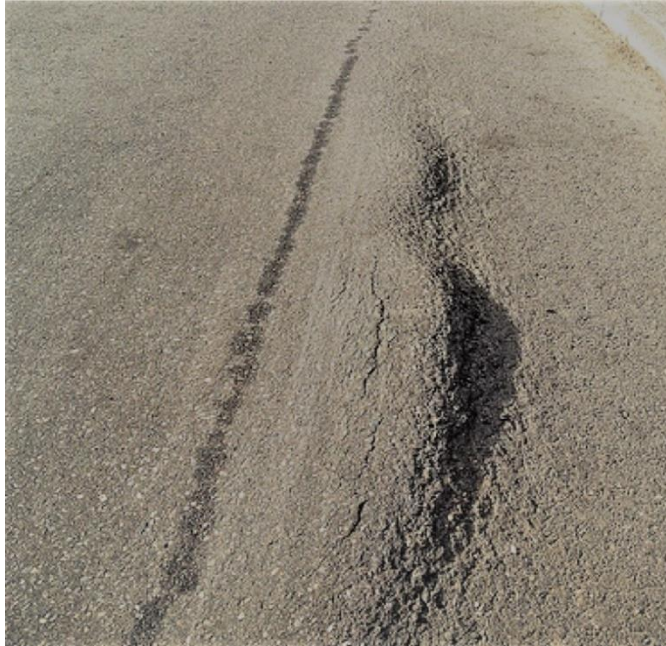
Figure 42: Shoving on road surface
