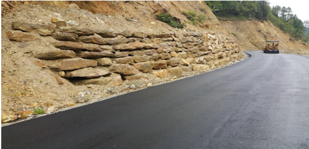
Boulder Wall – Innovative and effective drainage system
