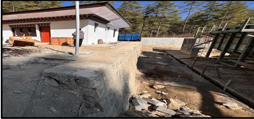
FIGURE 8: UNSAFE BREAST WALL HAS BEEN CORDONED OFF AND COMPLETED WITHOUT ANY SAFETY ISSUES
