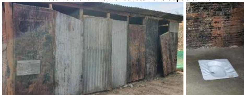
Photo 18 a & b. Worker toilets have septic tanks
