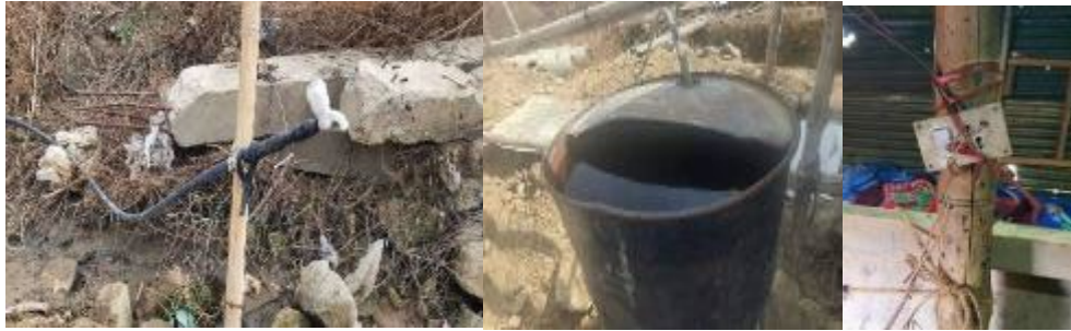
Photo 19 a, b & c. Tapped drinking water plus water storage for toilets and Electrical fixtures
