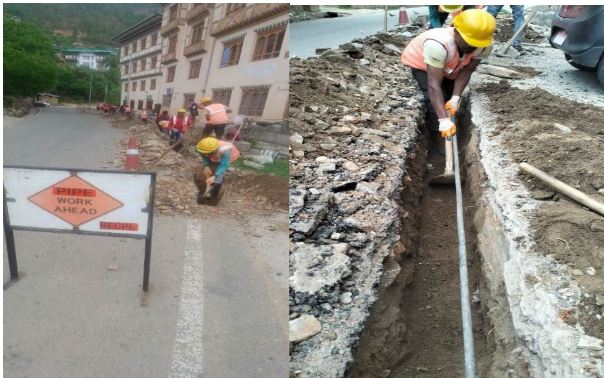
Photo 30 a & b. Barricade and safety signs employed while digging trenches with settlement areas.
