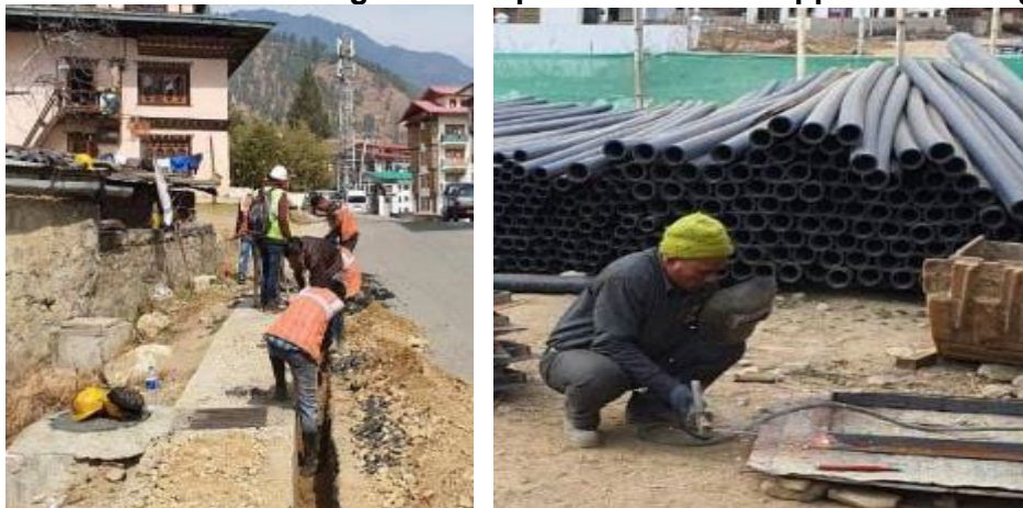
Photo 23 a & b. Worker using PPE camps and electrical appliances being used
