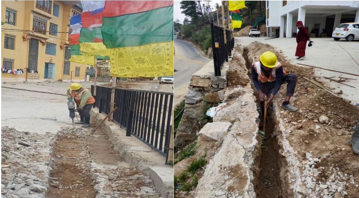
Photo 29 a & b. Manual digging of trenches to minimize the damages private properties.
