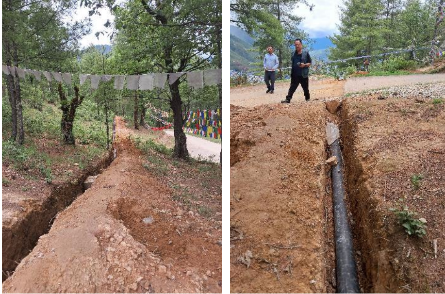
Photo 27 a & b. Completed trenches in the forest above the highway to Dechhencholing
