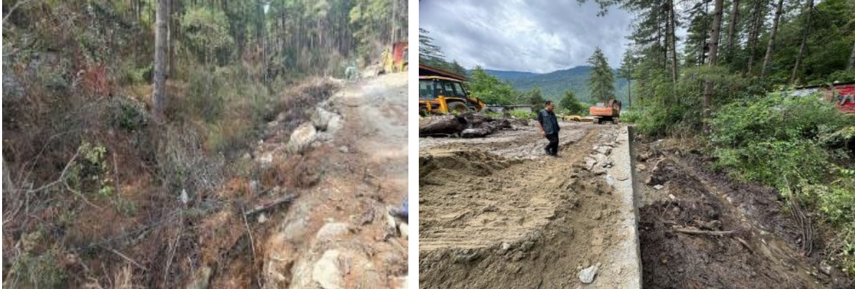
Photo 10 a and b - Clogged Drain and Retaining wall constructed and Drainage cleaned
