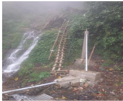
Pic-2: Water is drawn from a spring prone to landslides with exposed pipeline. To make climate resilient, there is a need to bury HDPE pipes and draw water from the secured source or apply water conservation measures to secure the water source of this type.
