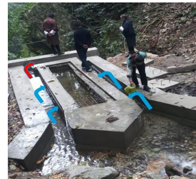
Pic-6: RCC filtration intake structure is a climate resilient technique to secure quality of drinking water
