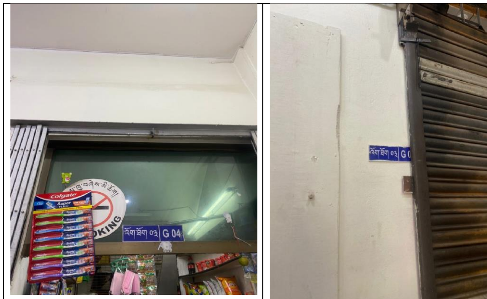
Figure 28 : Incorrect way to mount the number plates
